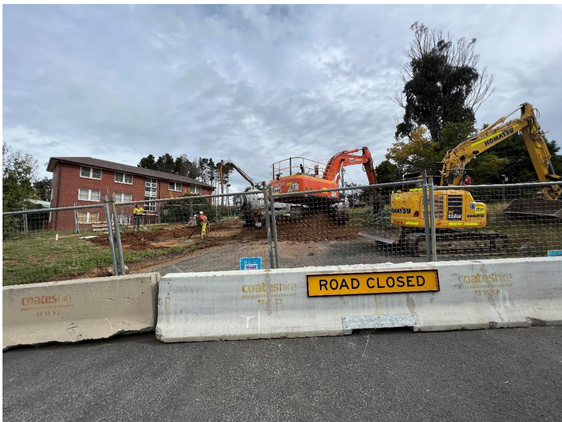
Solomon Lane is being upgraded to install utilities and connect services to Joule Ridge
